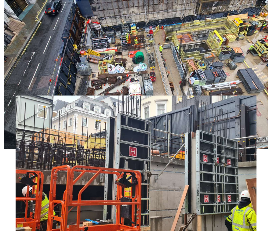
Zone 1 ground and garden level slab works, upstand walls and columns Looking towards Audley Square
