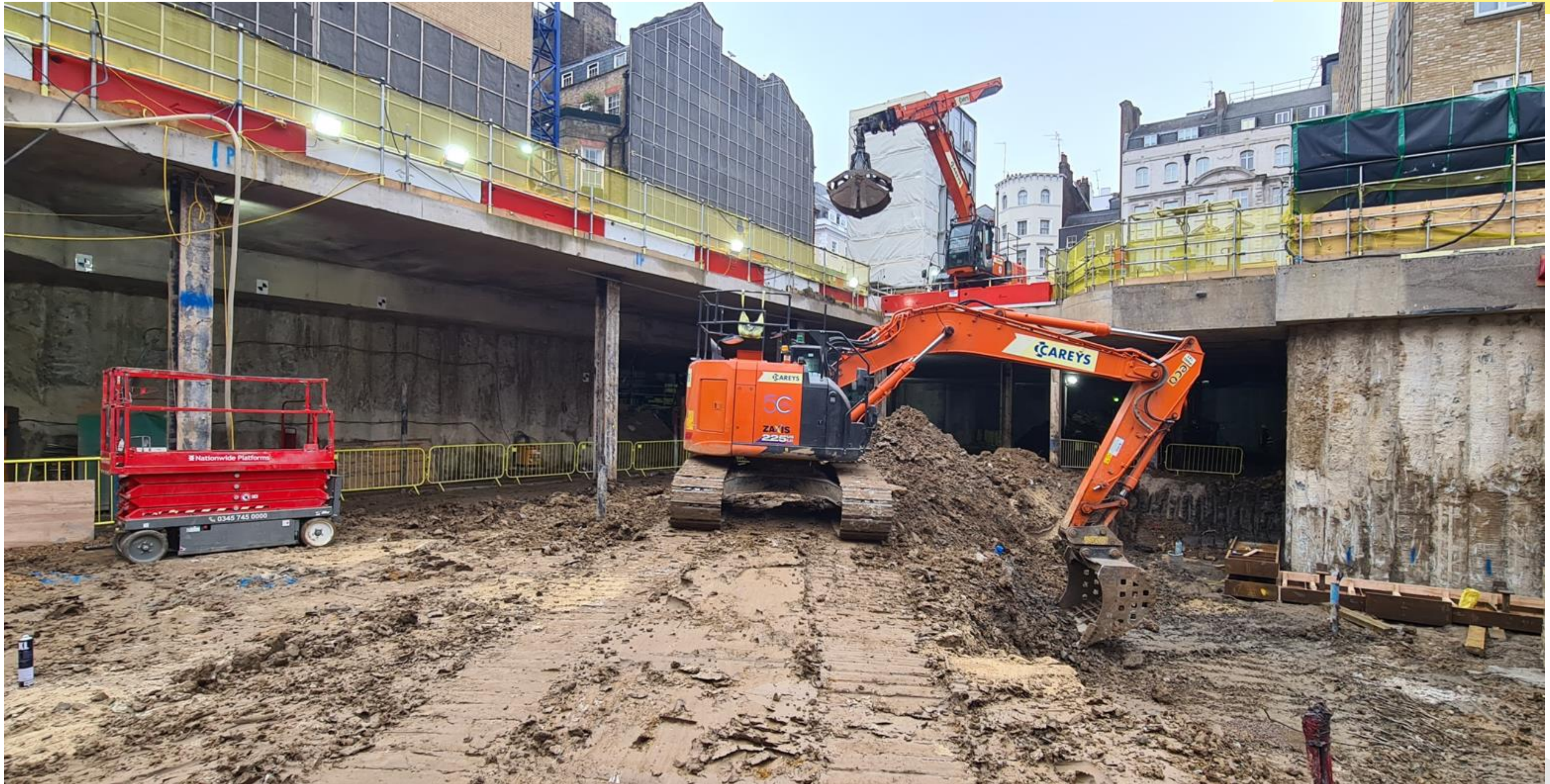
Long Reach Excavator Set Up on Garden Slab in Zone 1 – Removing Spoil to Tipper Trucks as part of bulk excavation works
