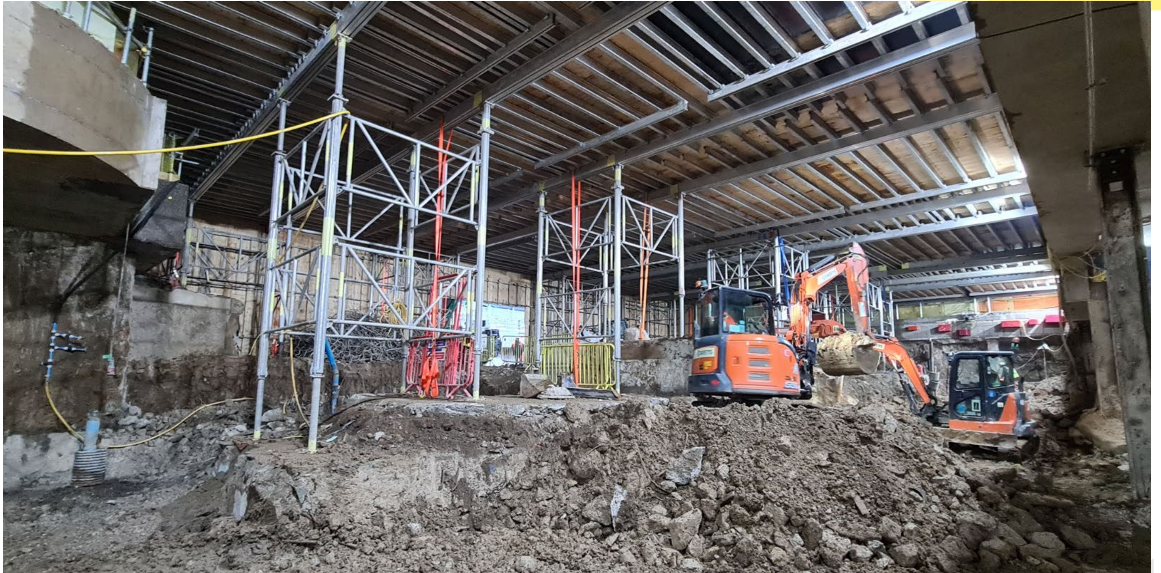
View from inside acoustic enclosure
