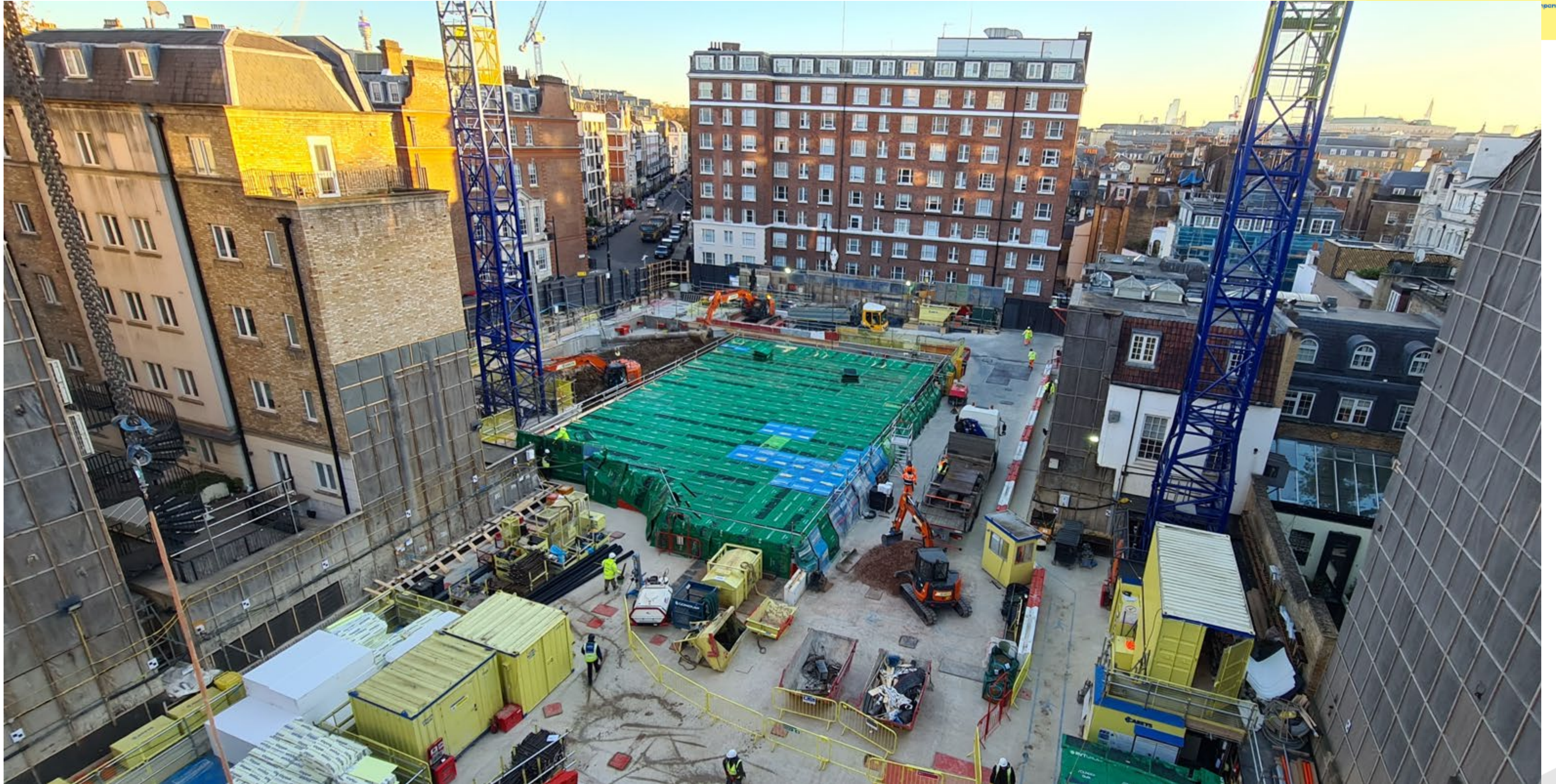
Slab removal taking place from inside the acoustic enclosure shown in Zone 2
