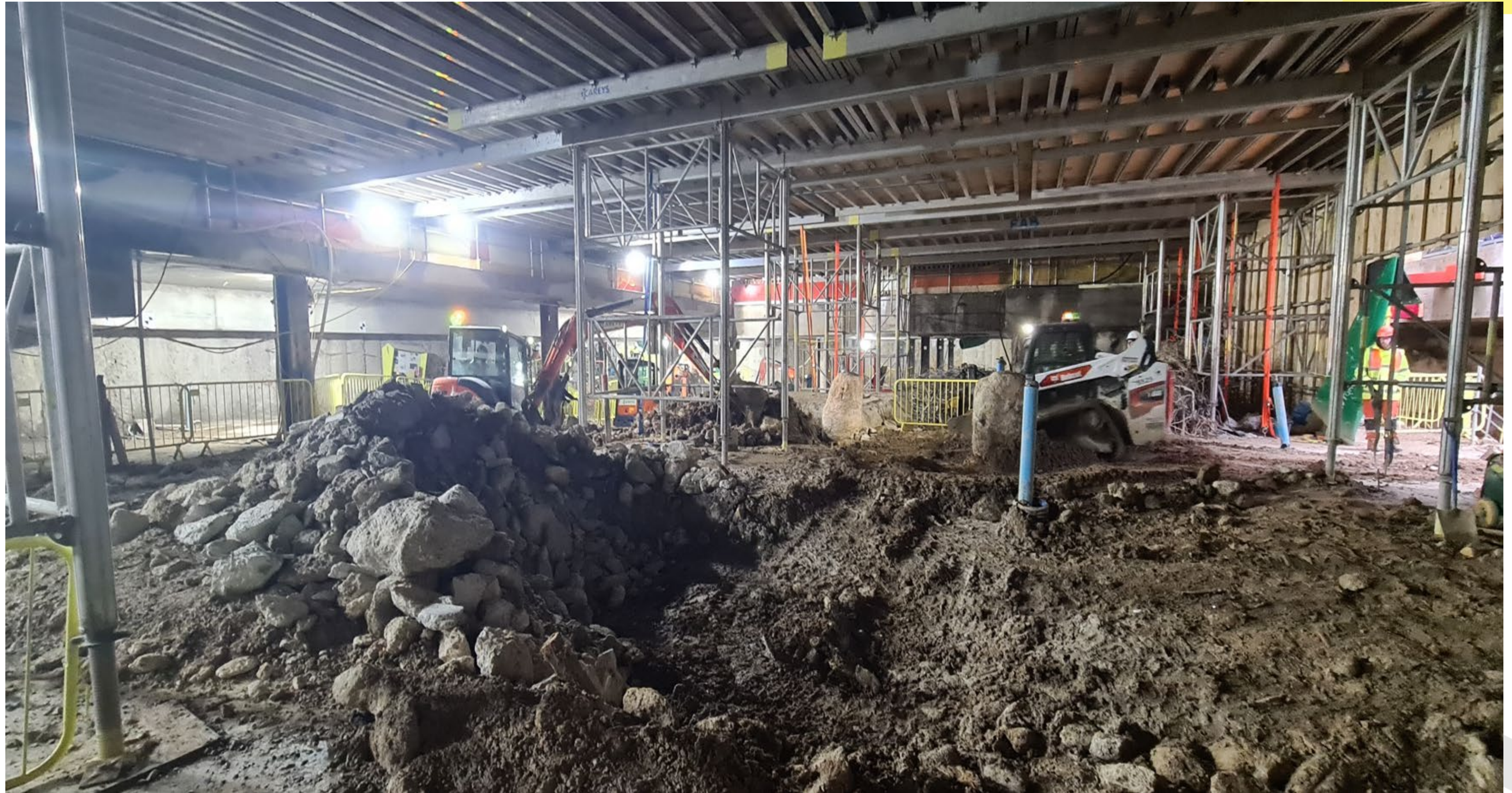
View from inside acoustic enclosure
