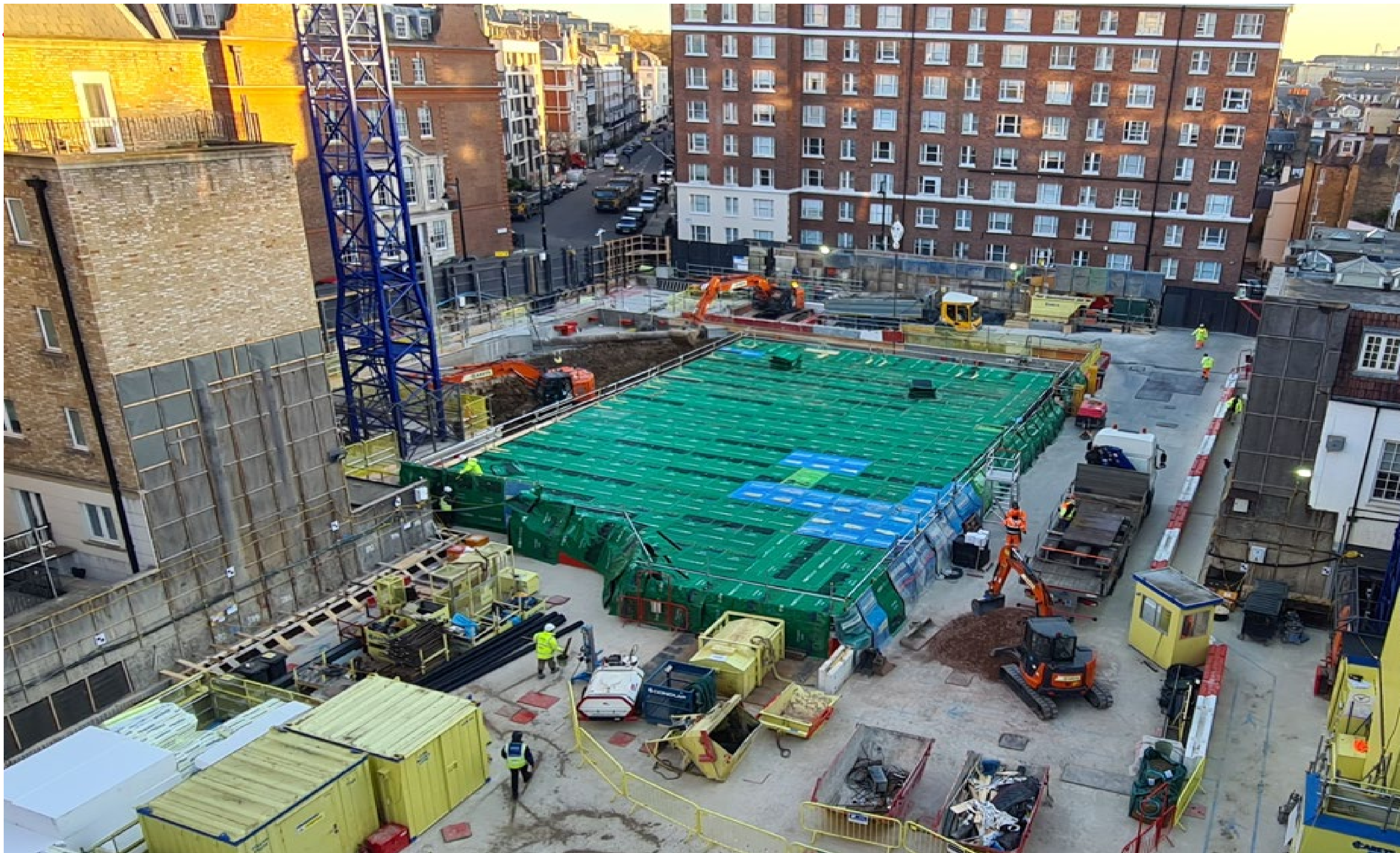
Acoustic Enclosure Frame – Zone 2
