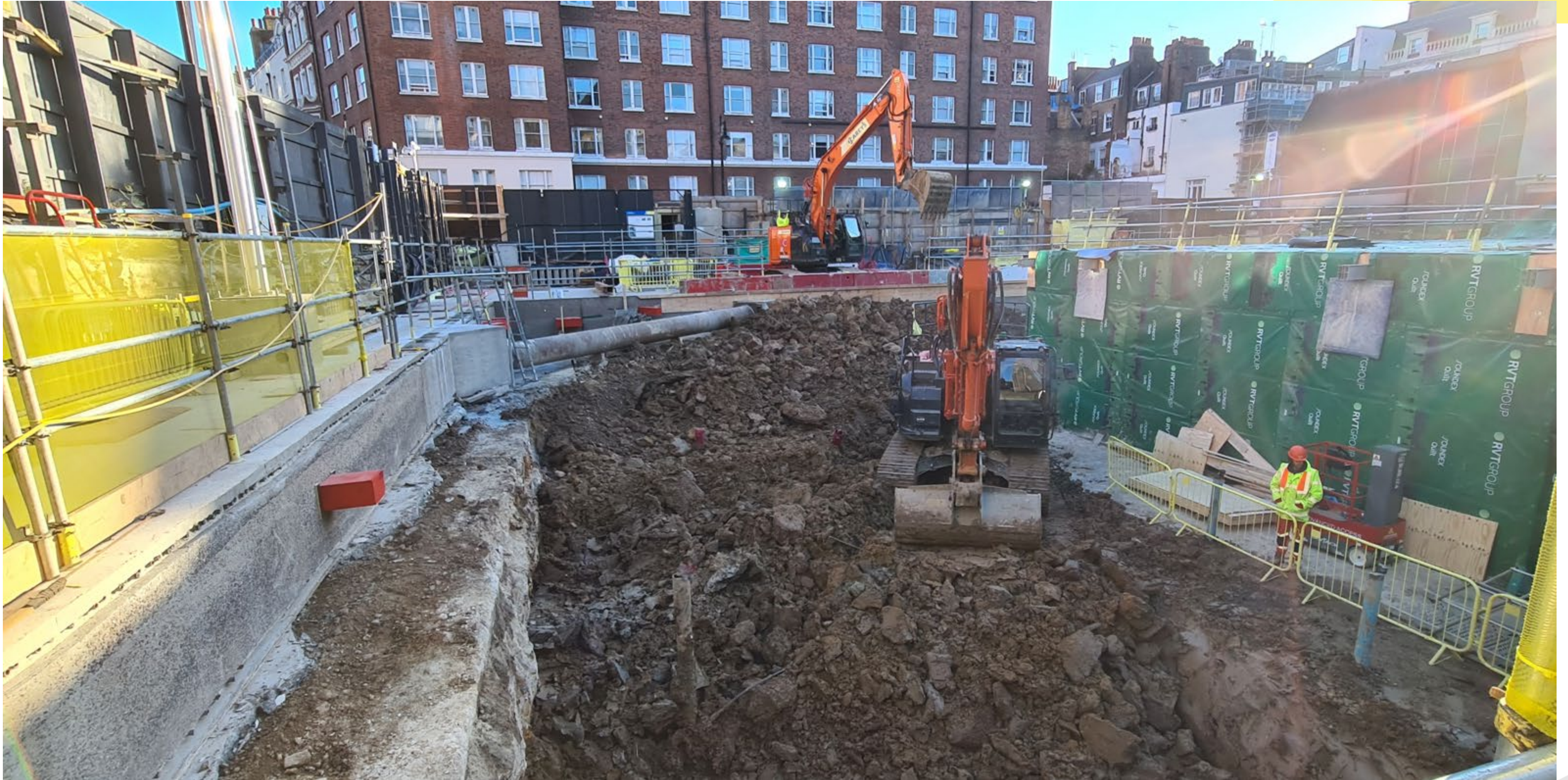
Excavator located on Garden Slab – Used to load tipper trucks for removal offsite
