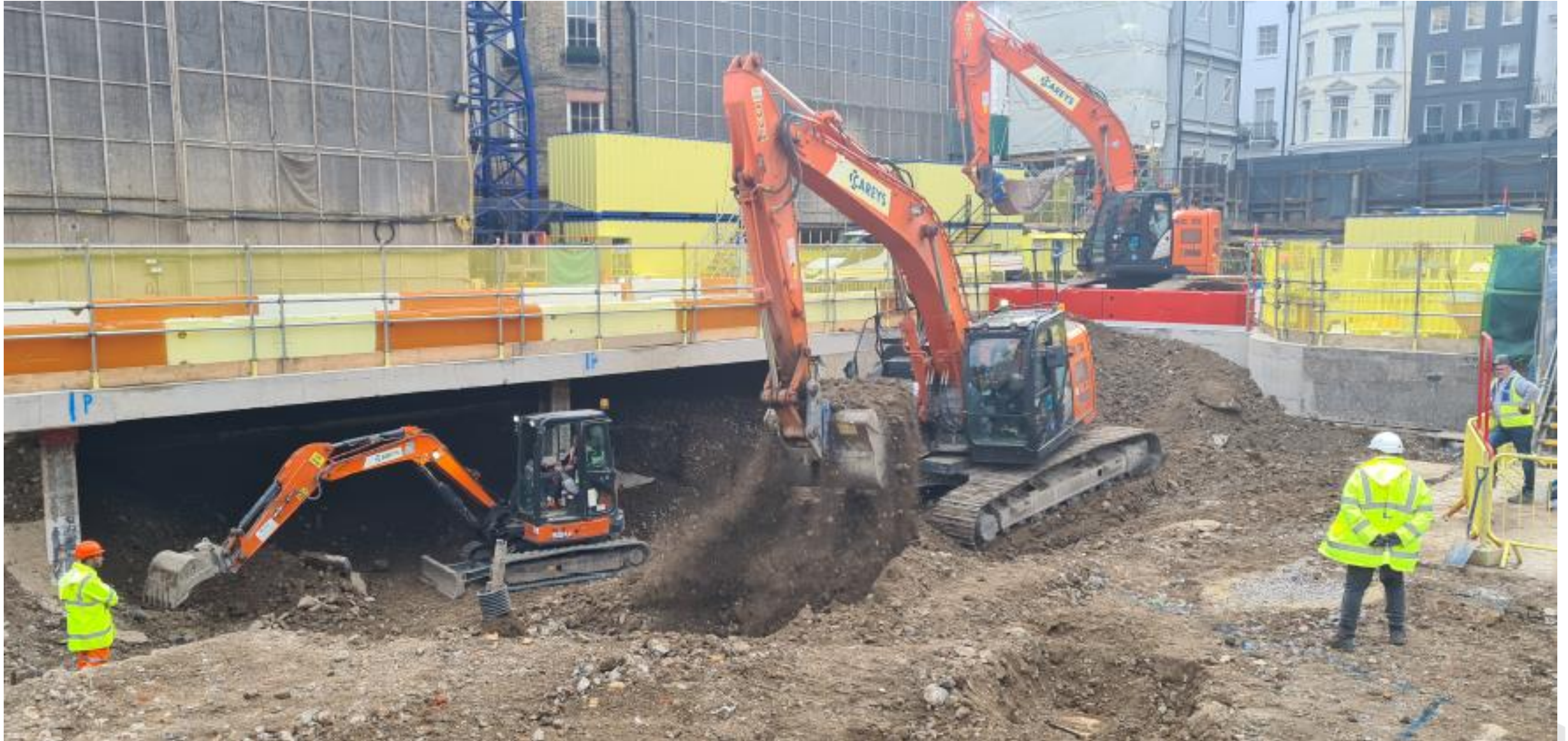
Typical View of Excavation Under The New Slab (Small excavator feeding larger excavator and stockpile)
