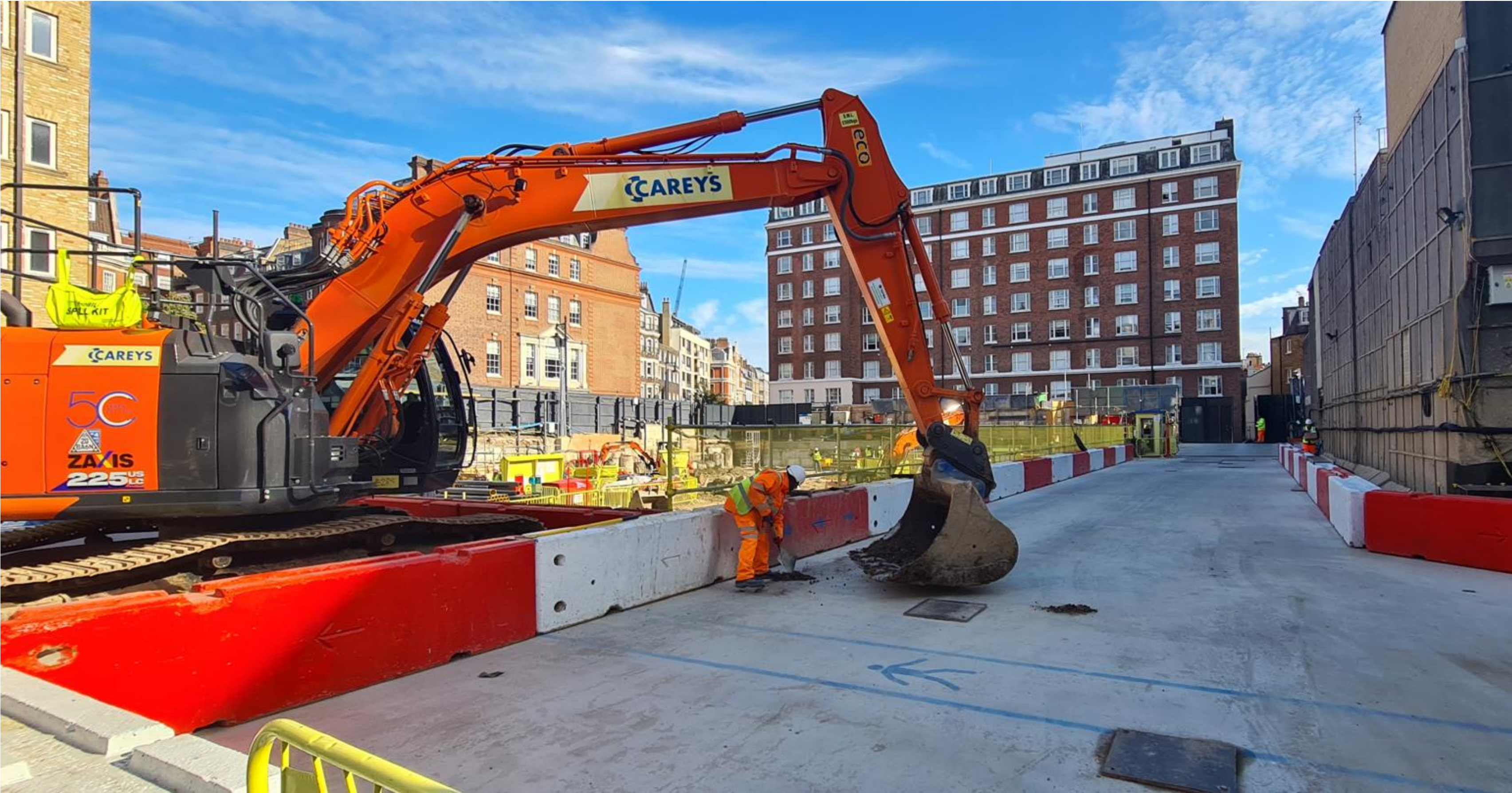
Excavator Set up on Garden Slab – Used to Remove Spoil From The Basement
