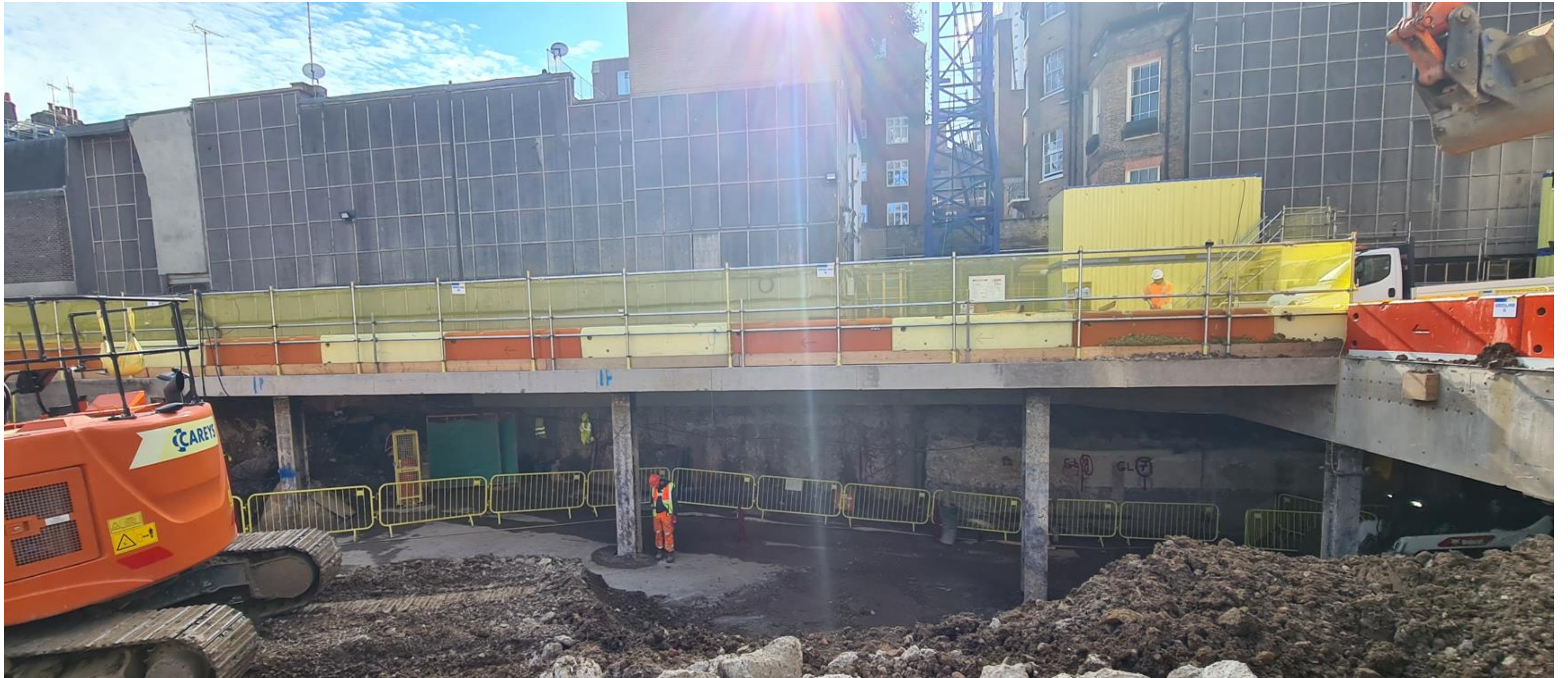
View into the basement area as excavation progresses (Looking in the direction of Red Lion Yard)
