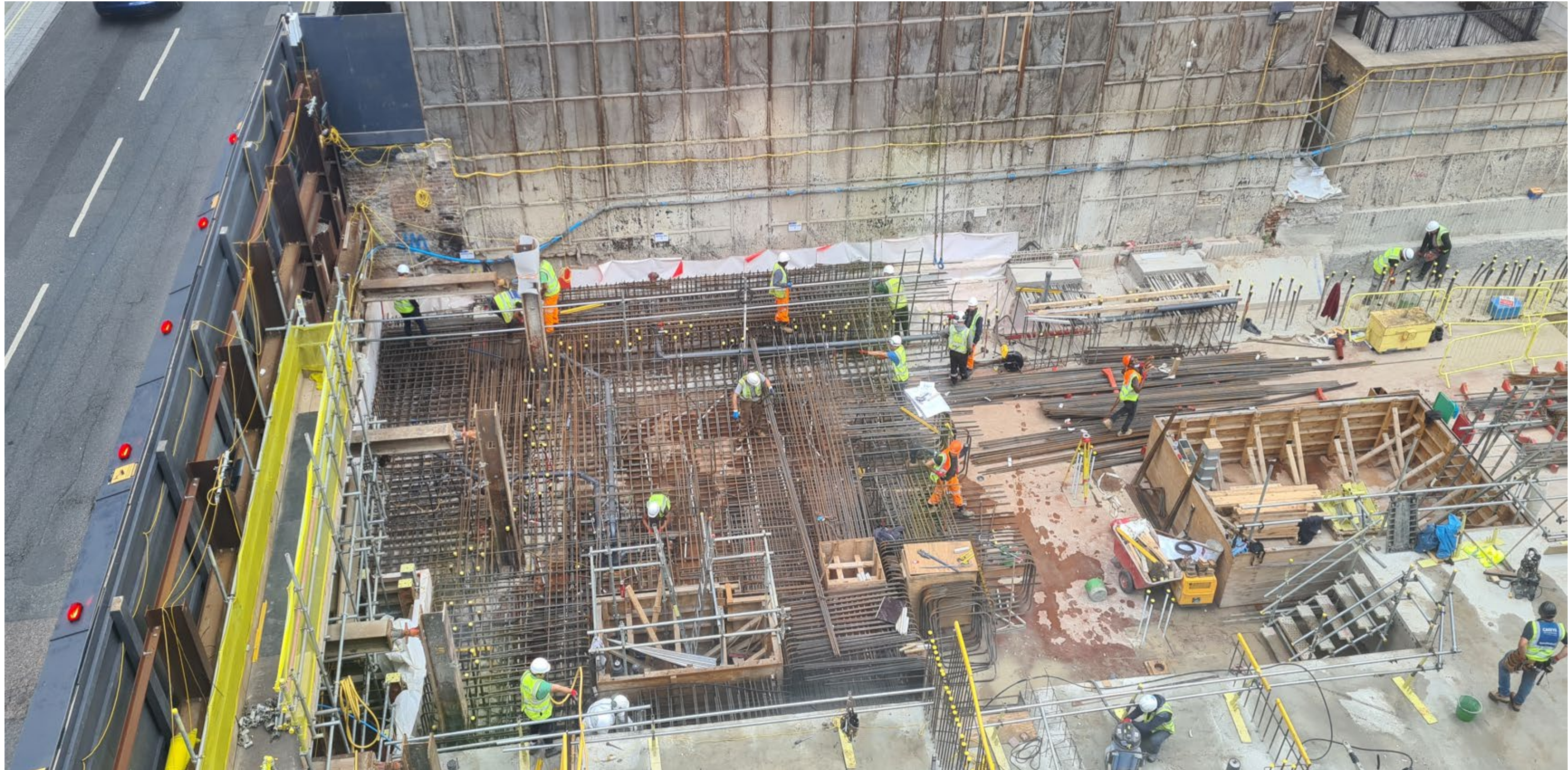
Typical plan view of steel fixing ongoing for slab construction beside the South Audley Street / Nehru Centre elevation
