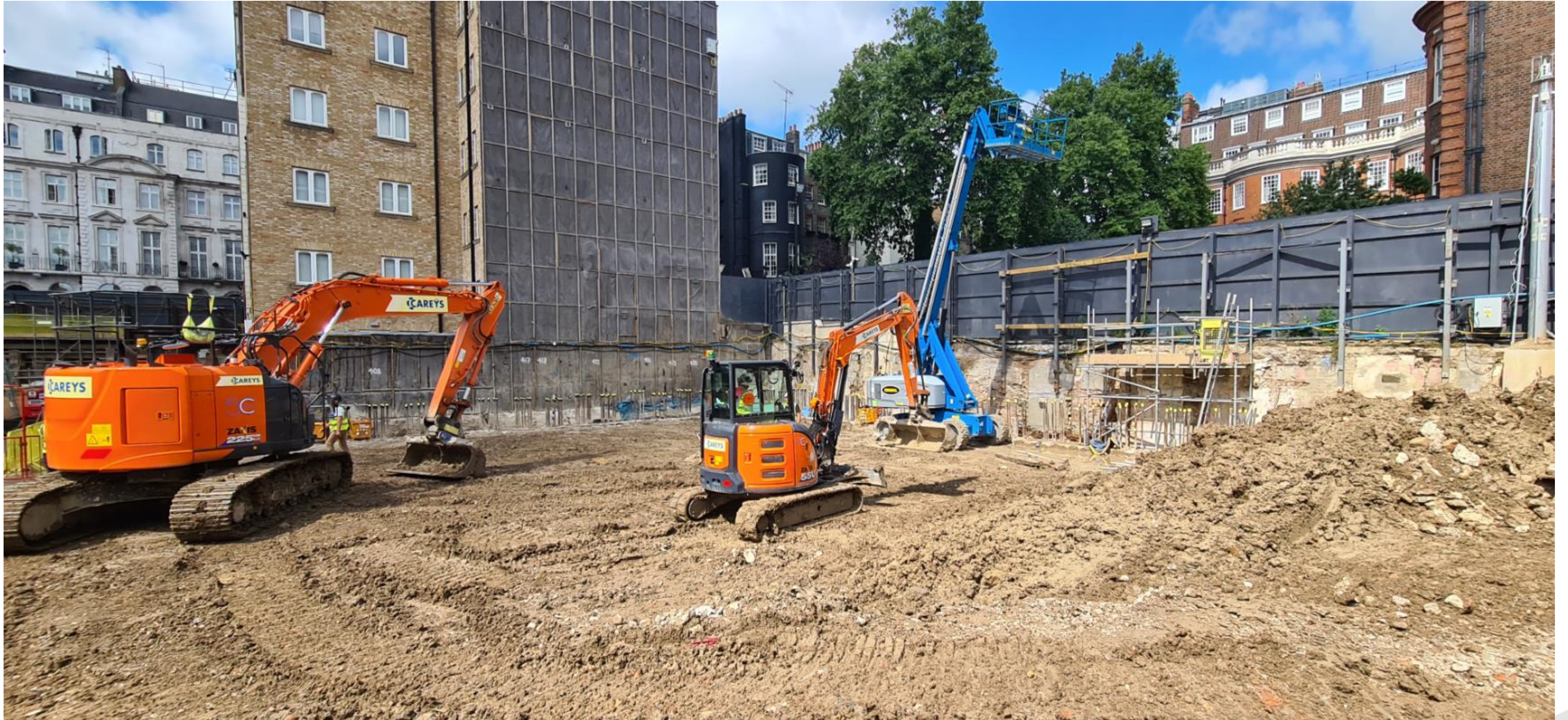
Groundworks ongoing in Zone 2 in preparation for slab construction. Machines grading the ground to the correct level.
