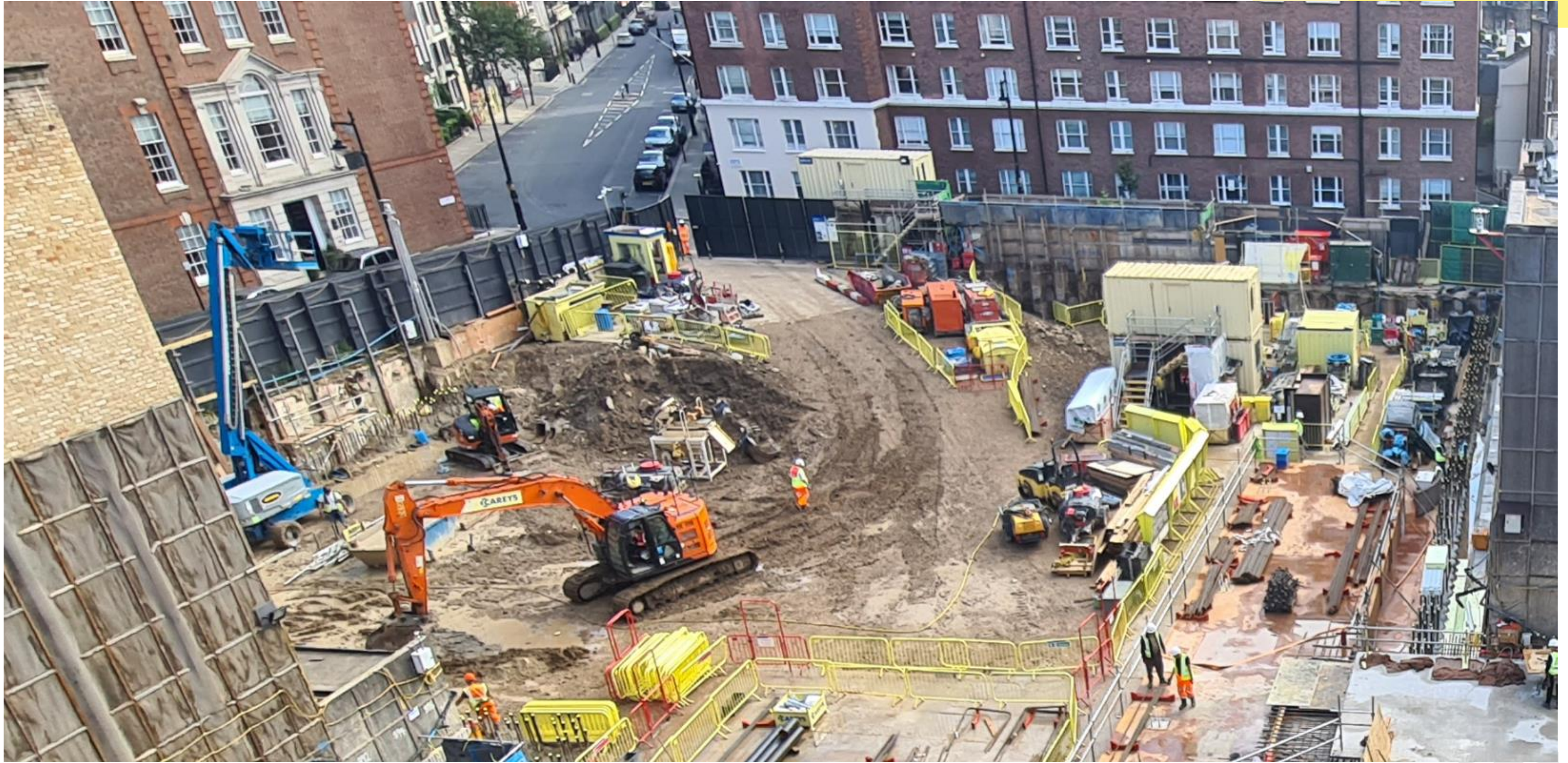
Groundworks ongoing in Zone 2 in preparation for slab construction. Vehicle access continues through Gate 2 on Waverton Street.
