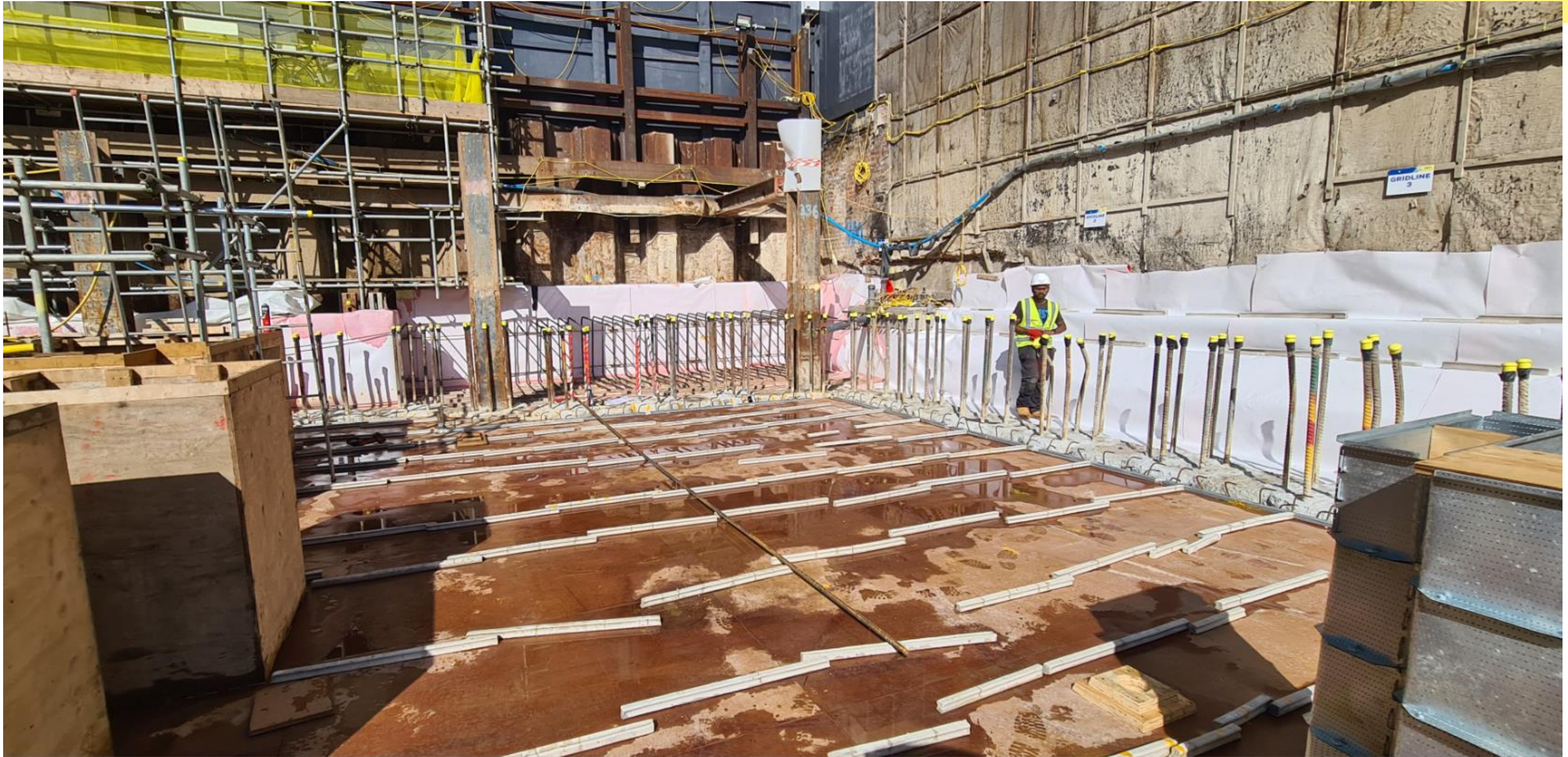
Steel fixing about to commence for slab construction along Nehru Centre elevation.
