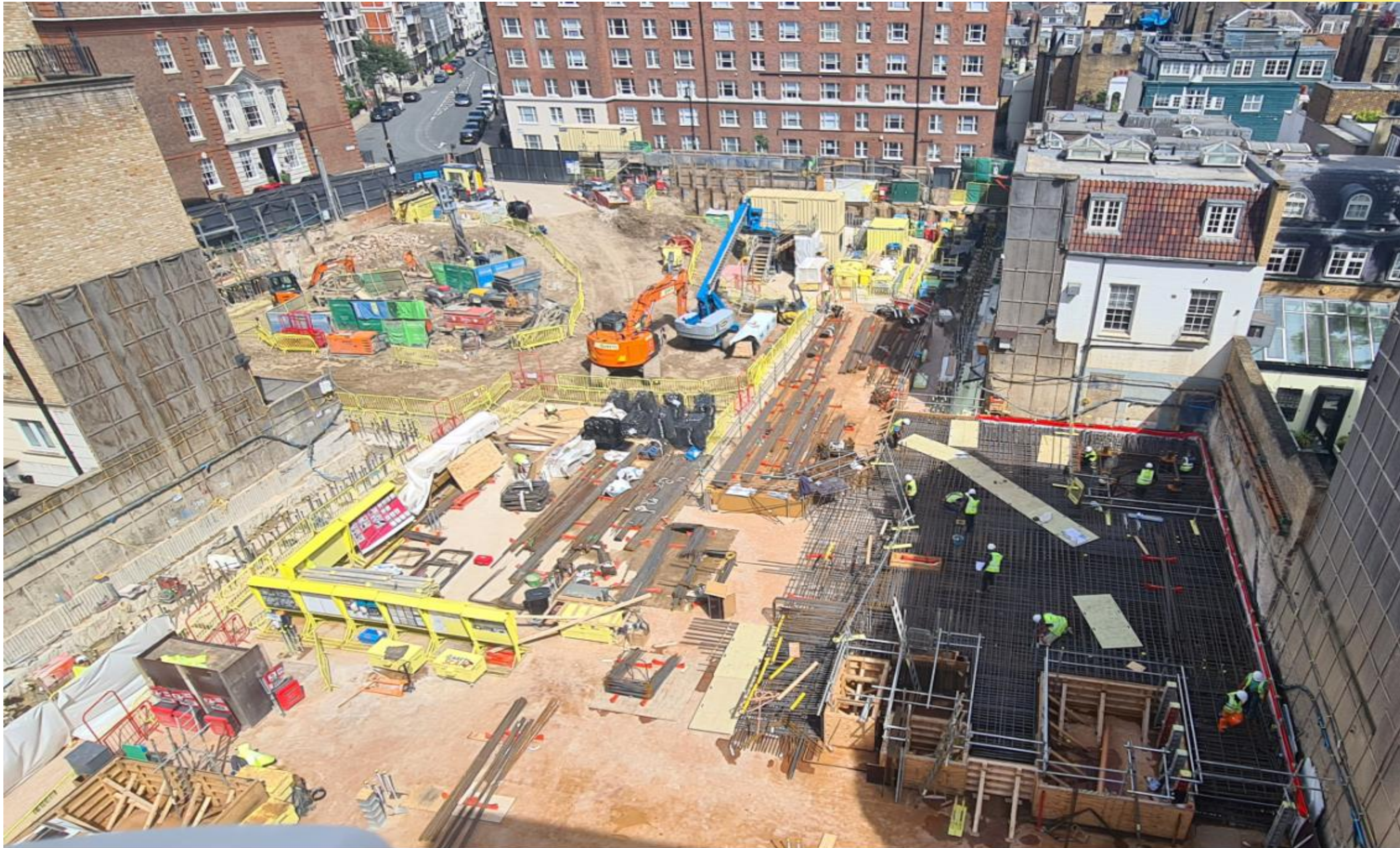
Typical plan view of slab formwork ready to receive concrete. (Location 3AS elevation)
