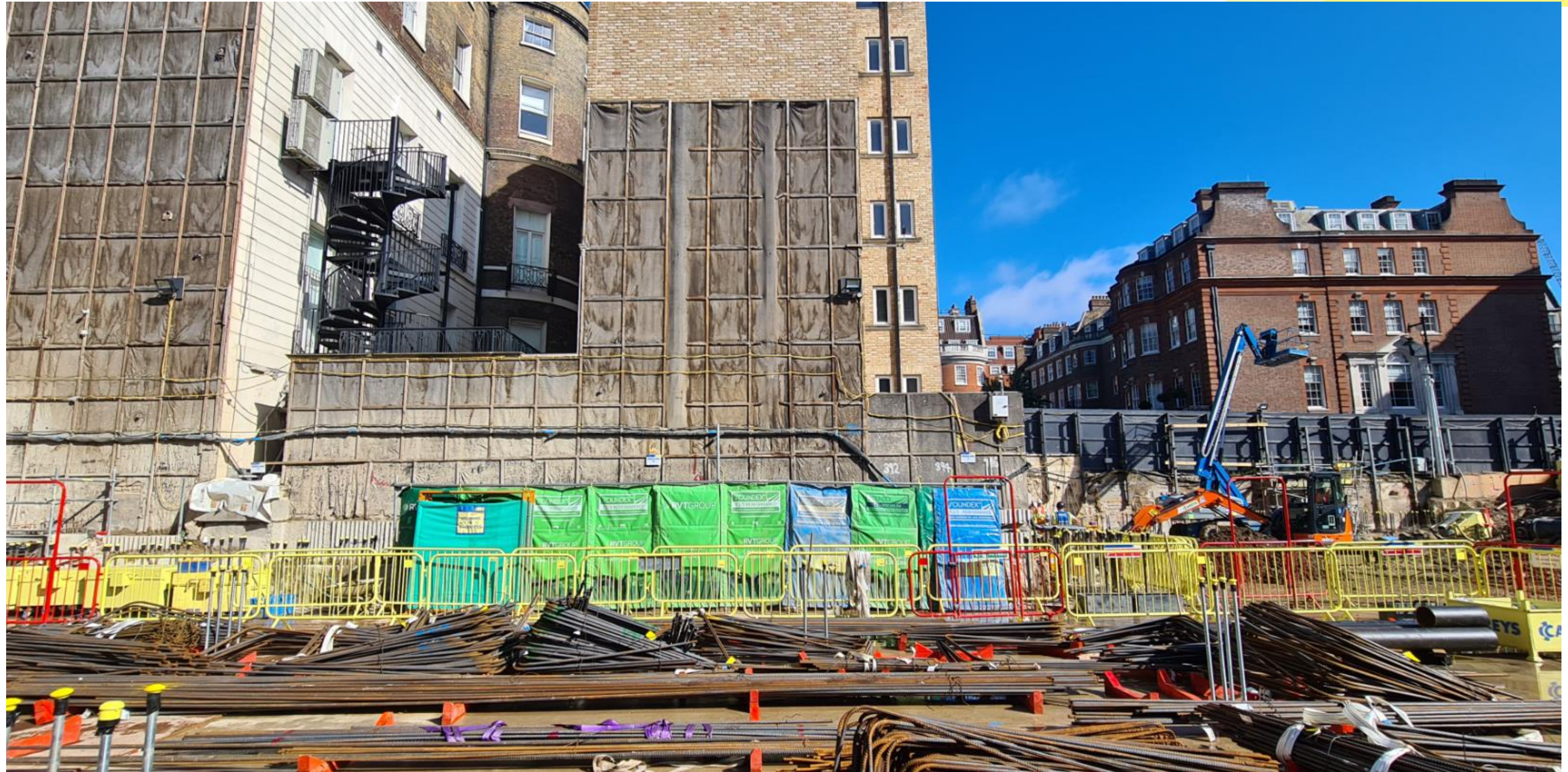
Typical example of concrete trimming works along 51 Hill Street elevation surrounded by acoustic noise barriers to reduce any potential noise.
