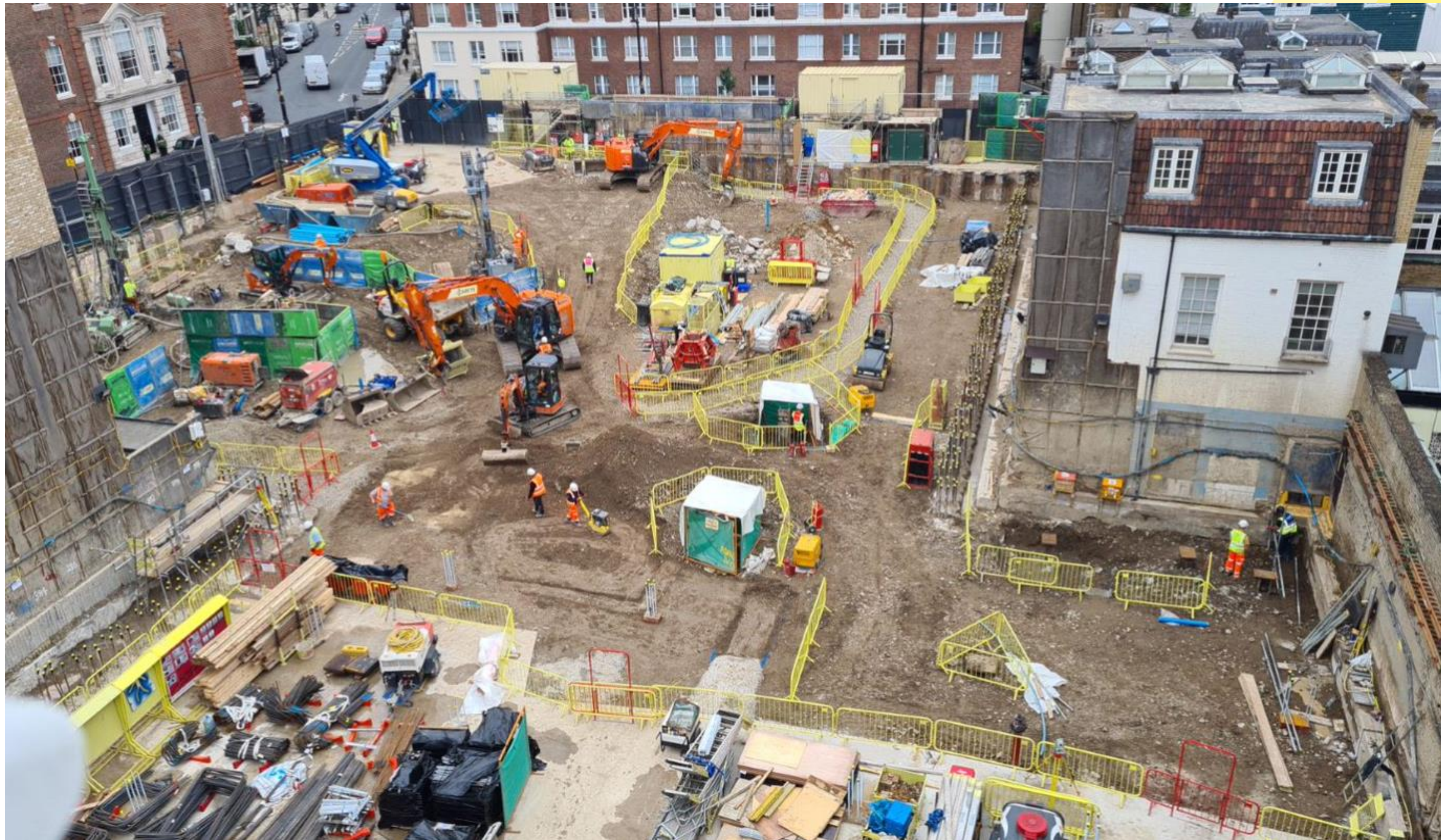
General Overview – Pile mat excavation complete to West of site. Ongoing excavation to East of site
