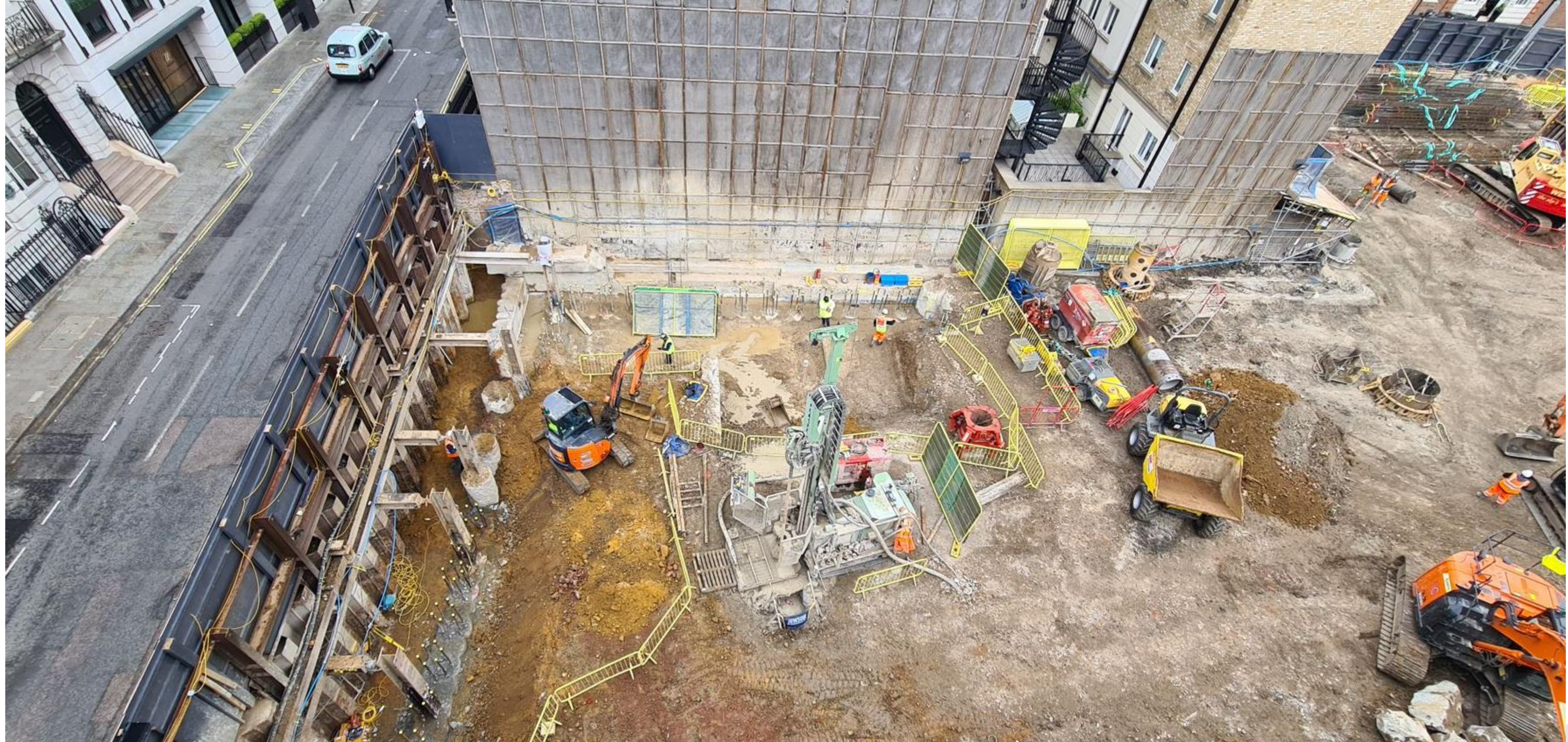
Typical Overview – Pilemat excavation from West to East across site in progress
