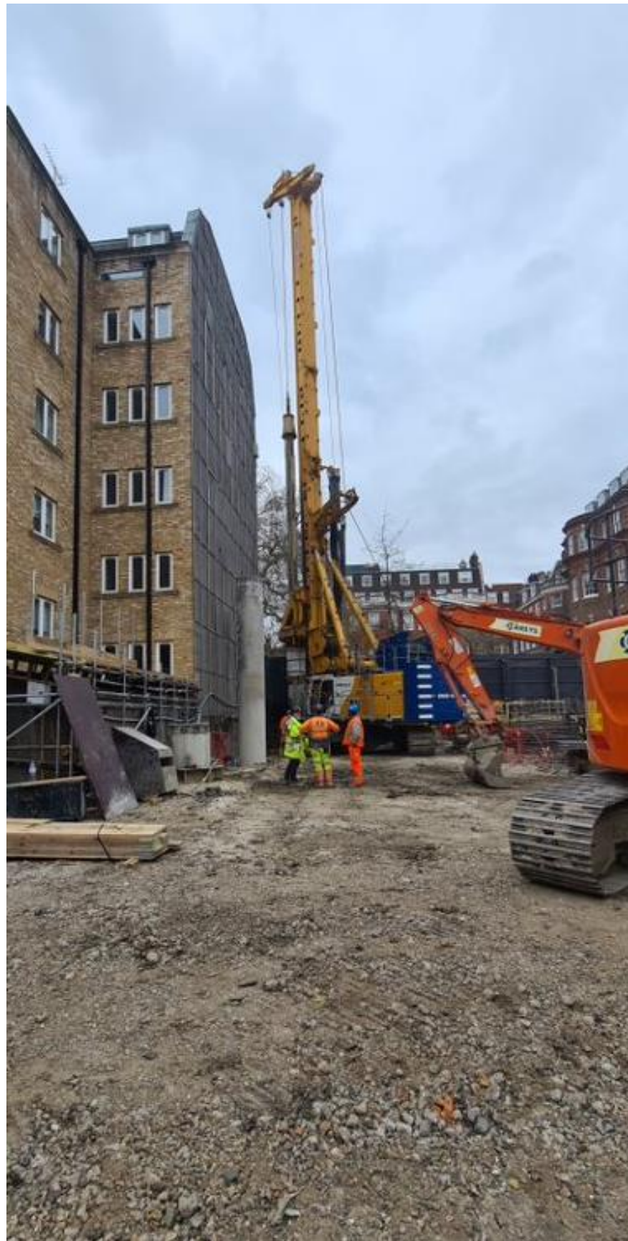
Rig – Installing New Perimeter Secant Piles To North of Site along Corner of 51 Hill Street
