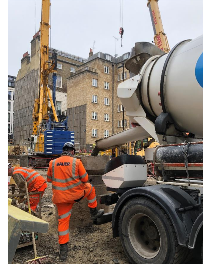
** (4) Pour Concrete through tremie pipe into the pile. Check and record concrete. (3 hrs)
