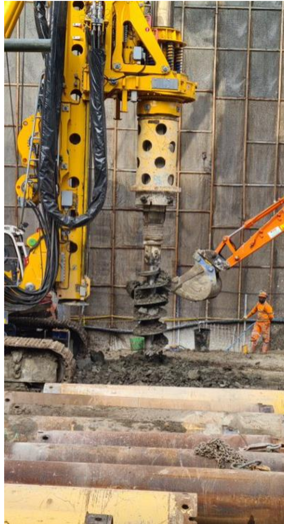
BPM – Use of Excavator Bucket Teeth To Remove Stubborn clay from auger
