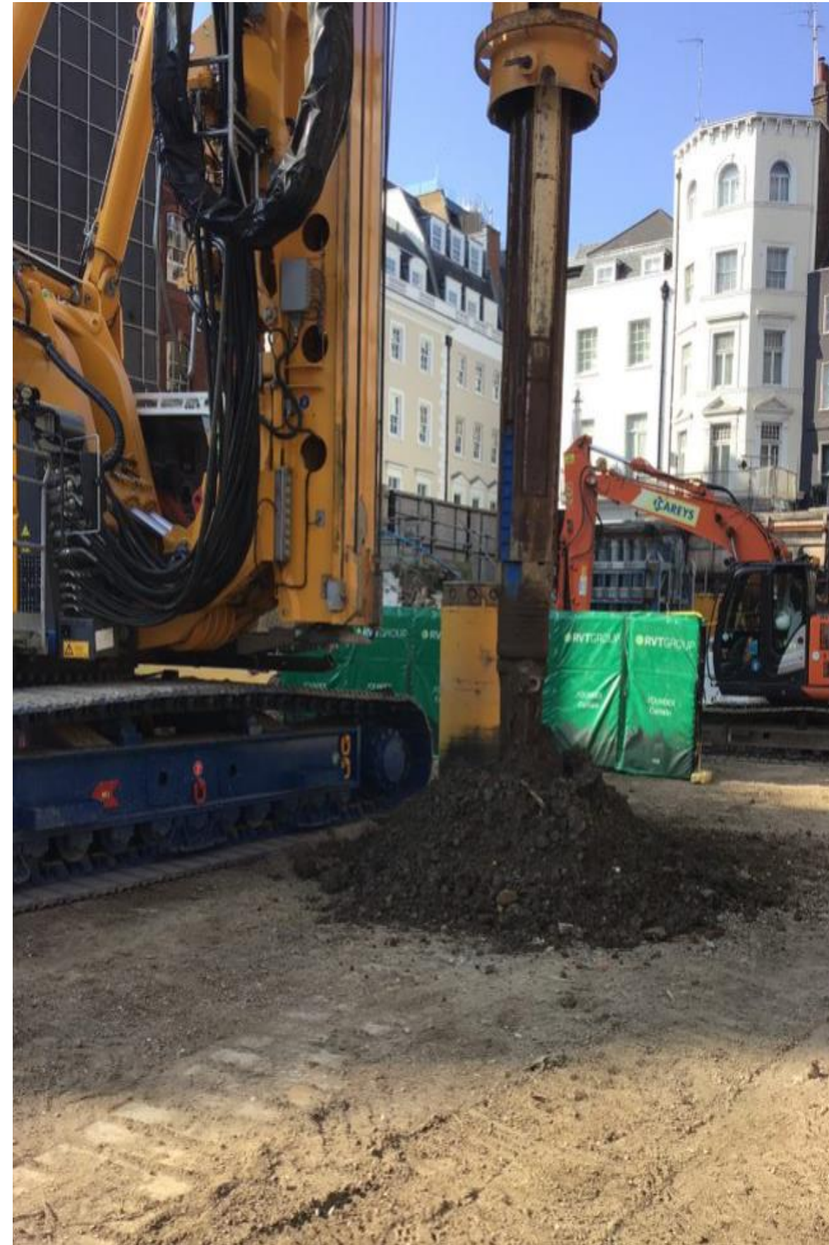
BPM – Spoil discharge, Spin into ground. Can only be used when safe to do so and no danger of hitting pipes in ground
