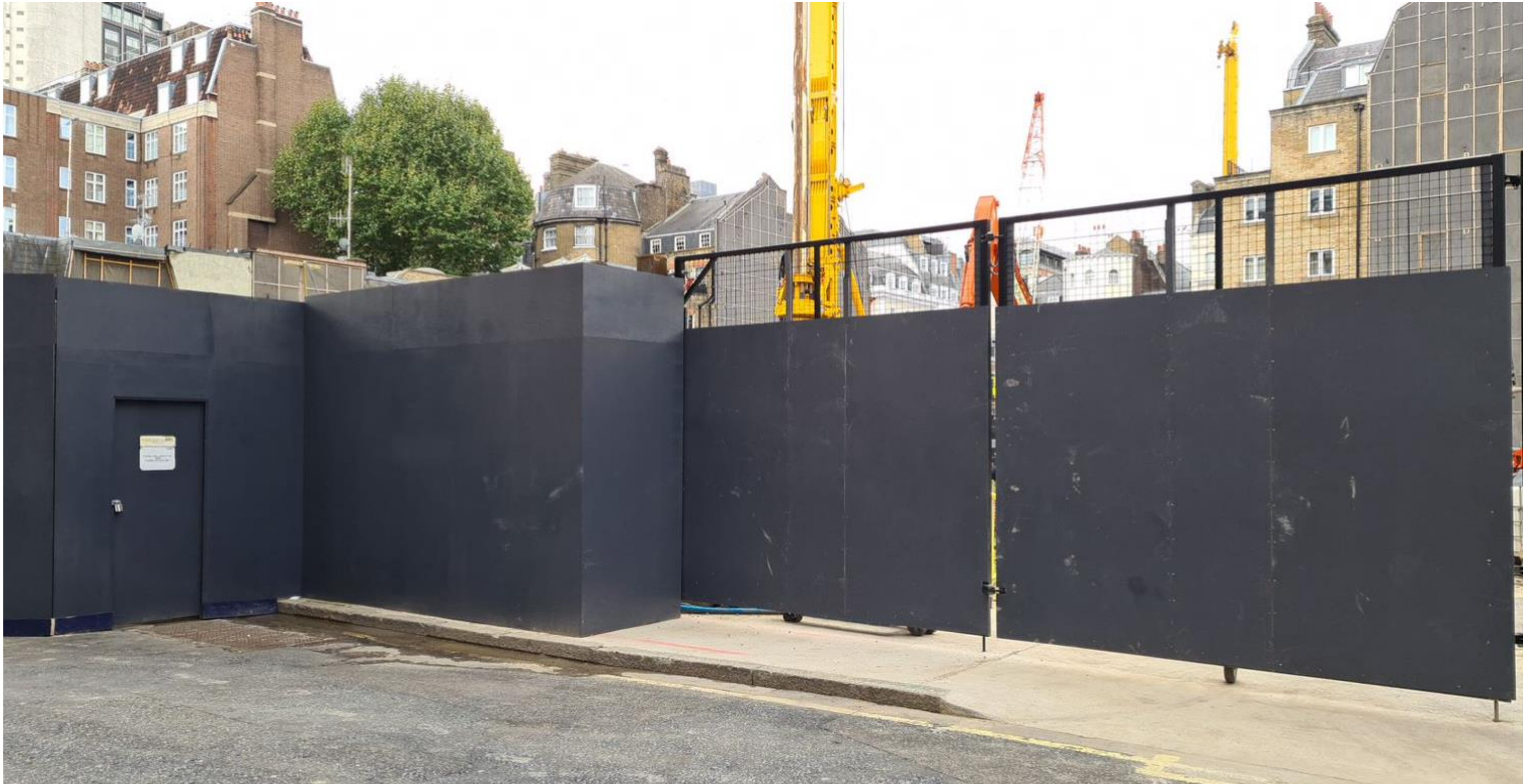
New Corner Access Gate Installed on Waverton Street – Keeping Traffic off Surrounding Streets
